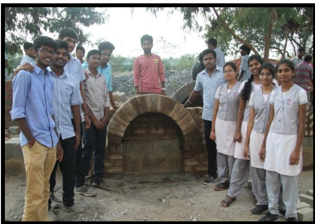
Construction of Arch by the Civil Engineering students on 03 rd February 2019 during the Hands on Training on “Brick Masonry Construction”
